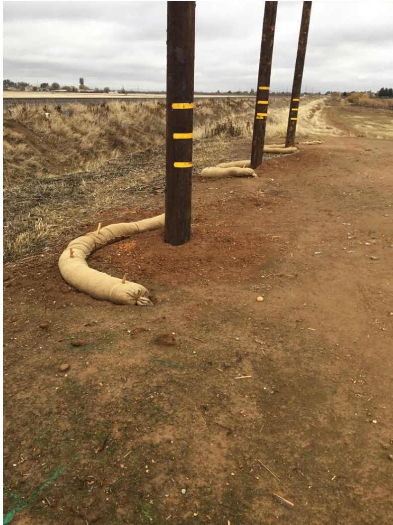
Photo 2: CPUC EM observed new installation of wattles around guard structures at structures 0/6 and 0/3 to prevent erosion in accordance with the SWPPP.
