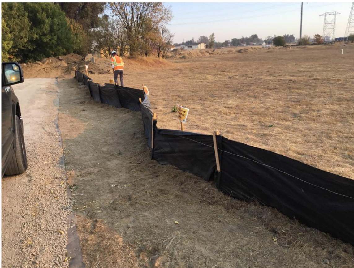
Photo 4: Sensitive environmental resources were clearly marked with signs and exclusion fencing at Landing Zone 0/1 in accordance with APM BIO-3. CPUC EM observed crews monitoring and maintaining the exclusion fencing onsite.
